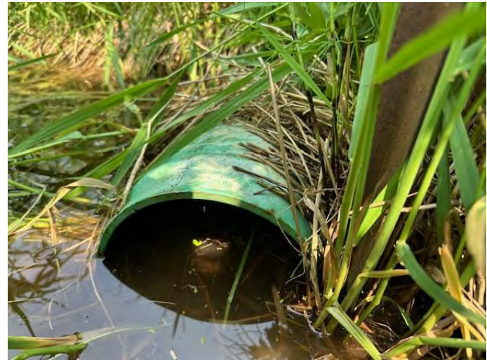
Partially submerged drainage outlet tiles at NAT-3 drainage ditch. No tolerance for increased water levels.
